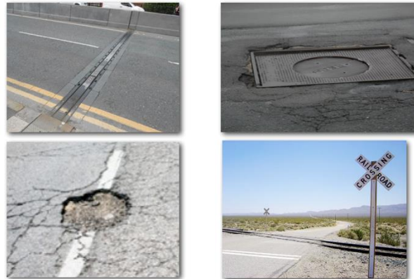
pothole v. not pothole
